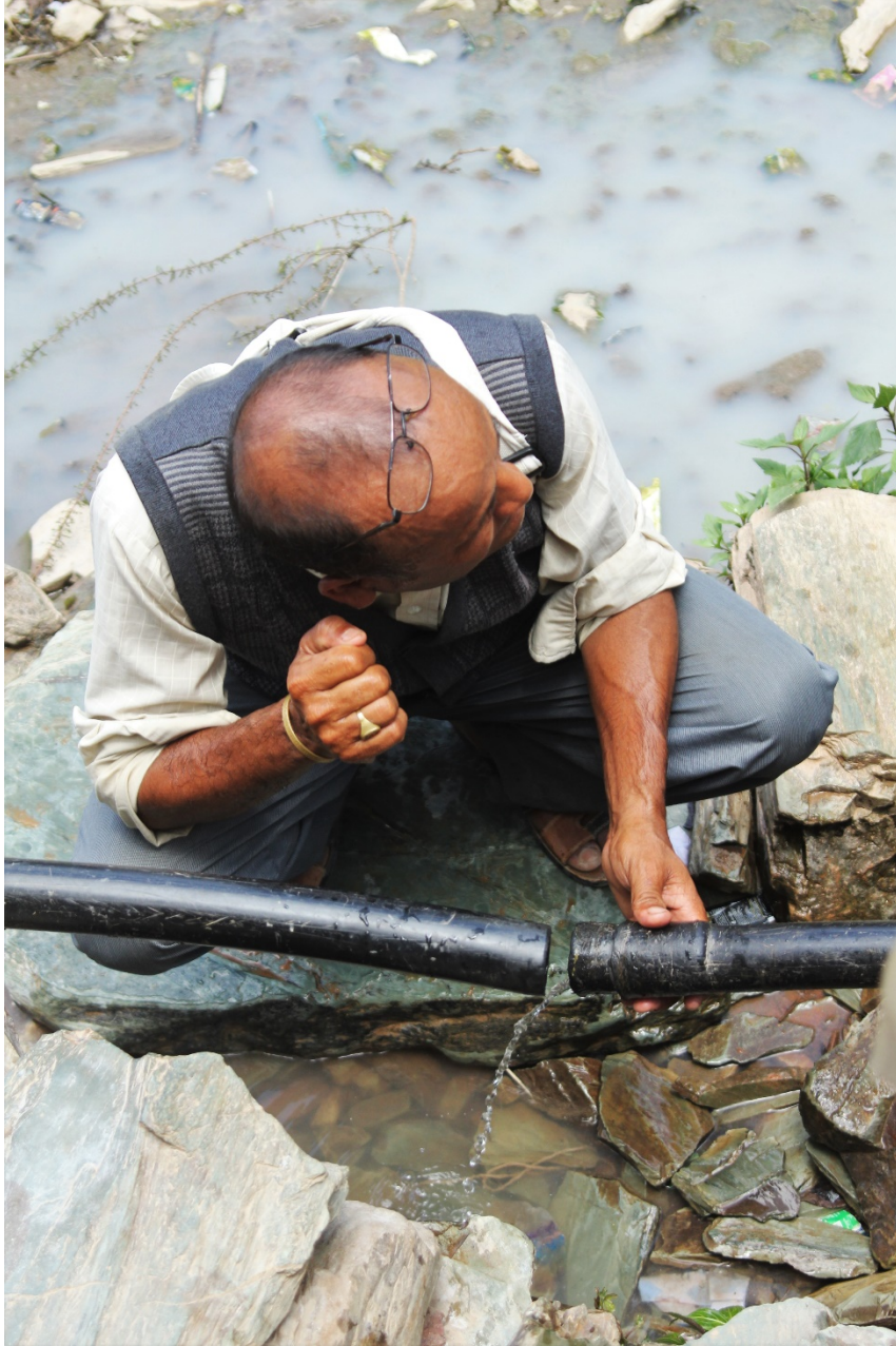
Figure 12: The black pipe which supplies water in Dumrikharka. Note how it lacks a tap and first be separated to access the water.
